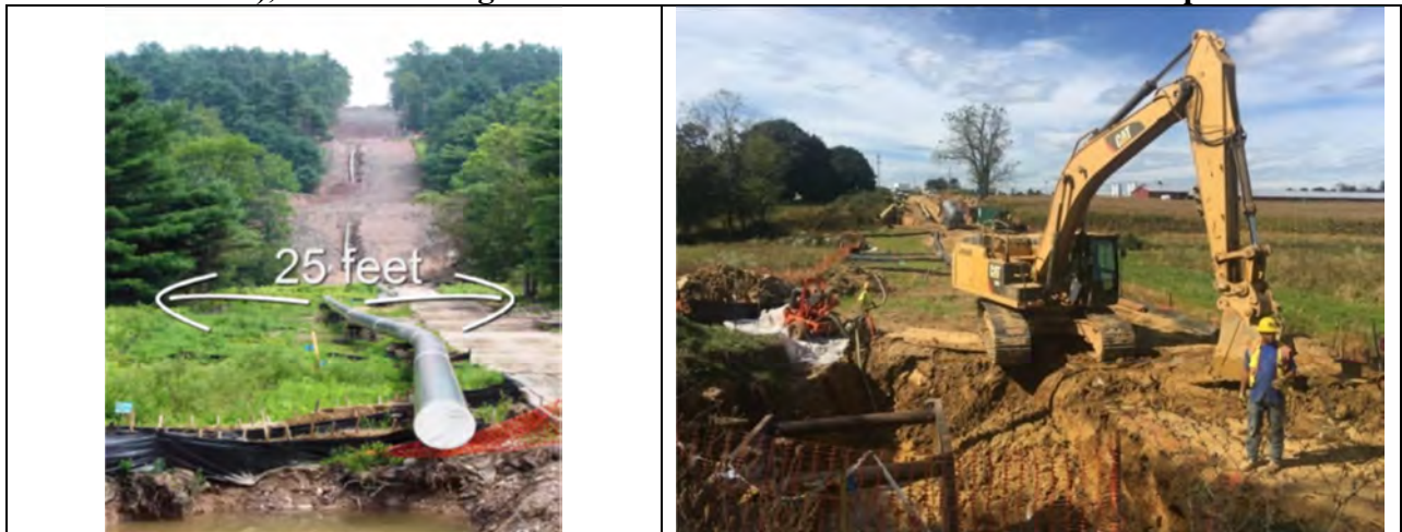
Figures 6a and 6b. Typical Pennsylvania 15-meter pipeline RoW (25 feet on either side of centerline), 84 and clearing of RoW for 20-inch diameter Mariner East Pipeline 85
